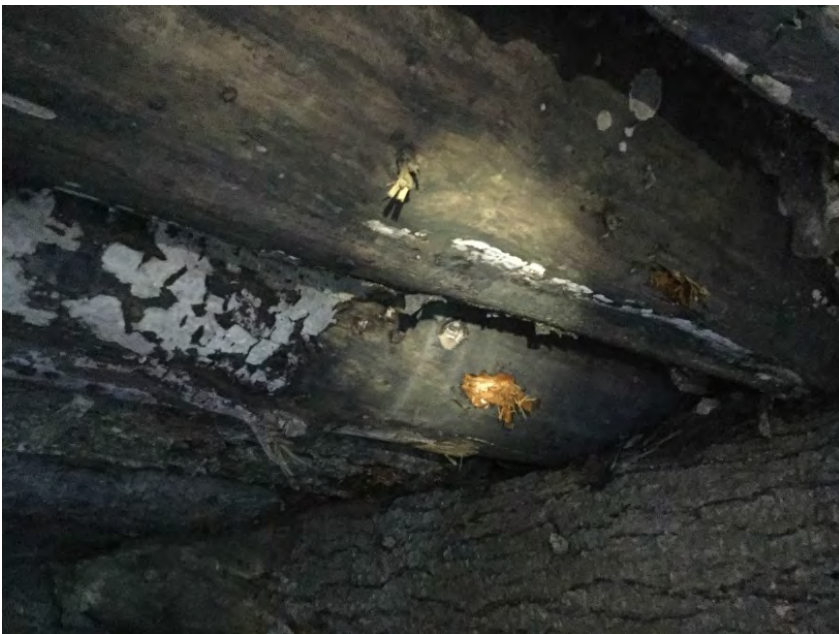
Stringer 2 & 3 Fungal Growth
