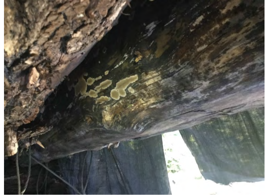
Stringer 14 Fungal Growth
