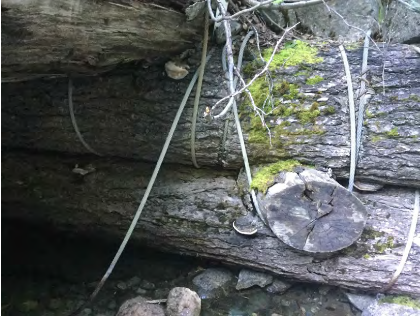
Right Abutment Fungal Growth
